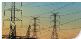
Newman HV Power System
