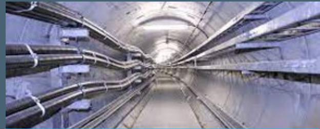
Sydney CBD 132kV Cable Tunnel
